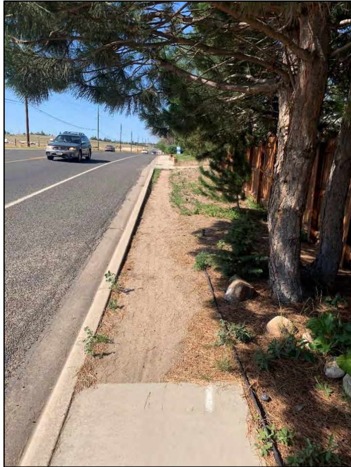
Figure 2-G Missing sidewalk on Powderhouse Road
