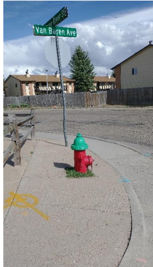
Photo 2 Substandard sidewalks and ADA corners
