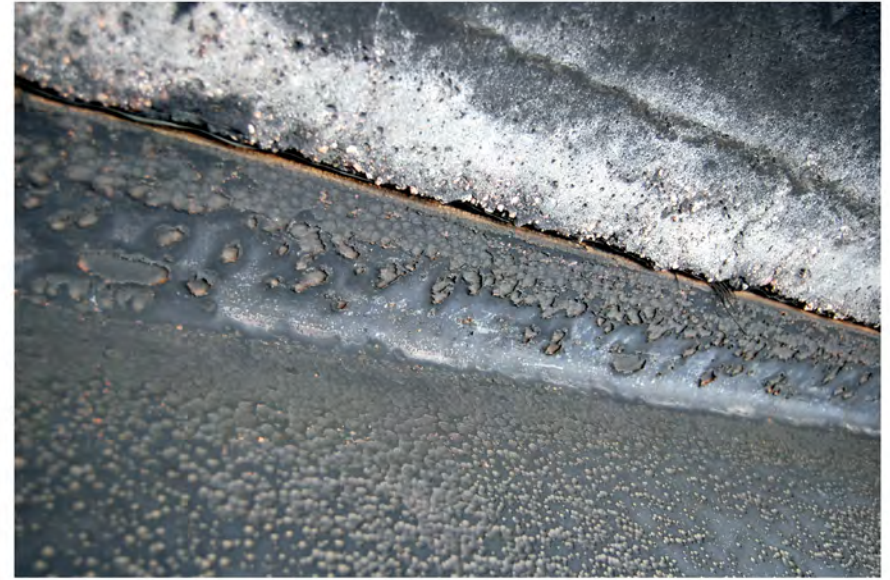
RUST PITTING OF TOP FLANGE AND WEB
