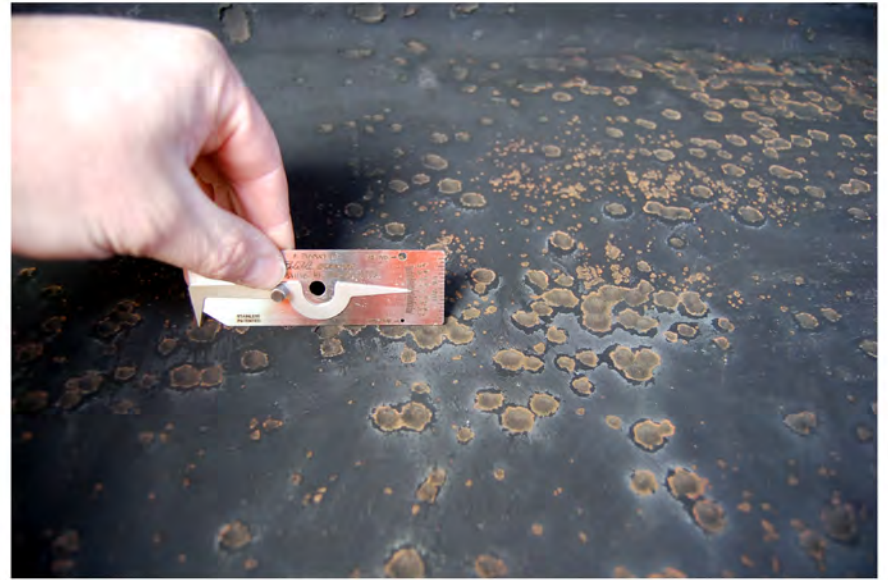
GIRDER PITTING MEASURE 1/16" DEEP
