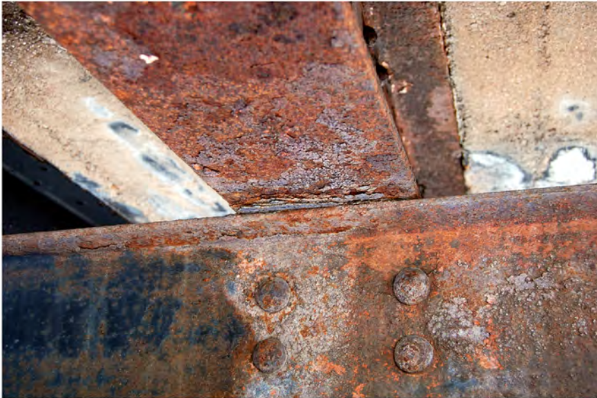
PACK RUST AT GIRDER/CAP CONNECTION
