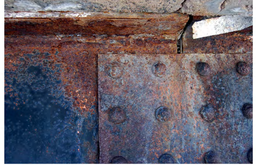
RUST W/SECTION LOSS TO GIRDER ENDS UNDER DECK JOINT
