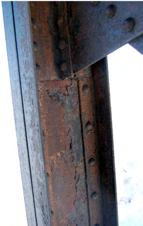
RUST W/SECTION LOSS AT TOP OF STEEL COLUMN
