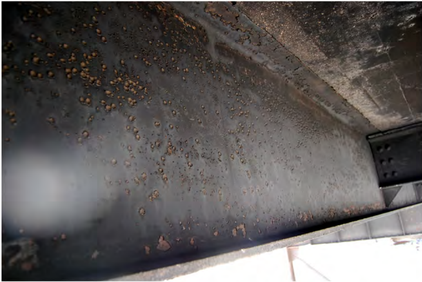
PITTING OF CENTER SPAN GIRDER
