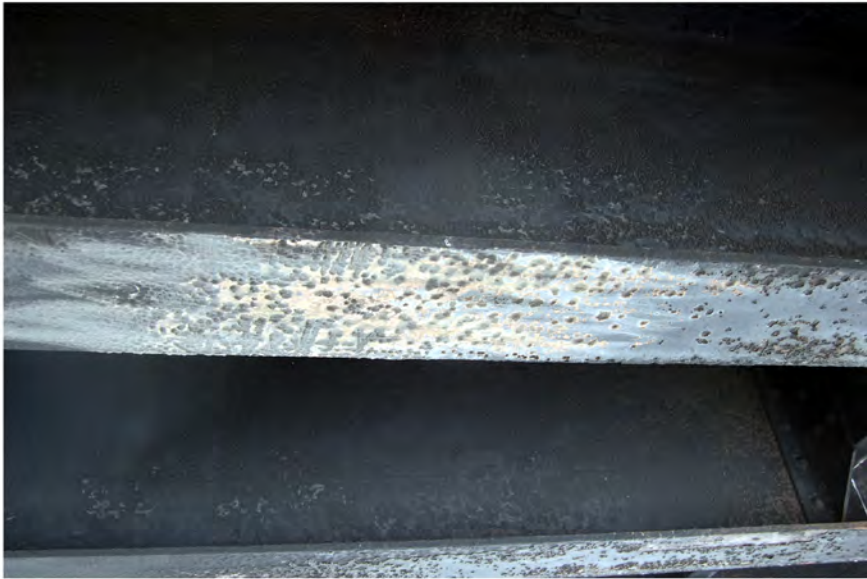
RUST PITTING ON BOTTOM FLANGE OF CENTER SPAN GIRDERS
