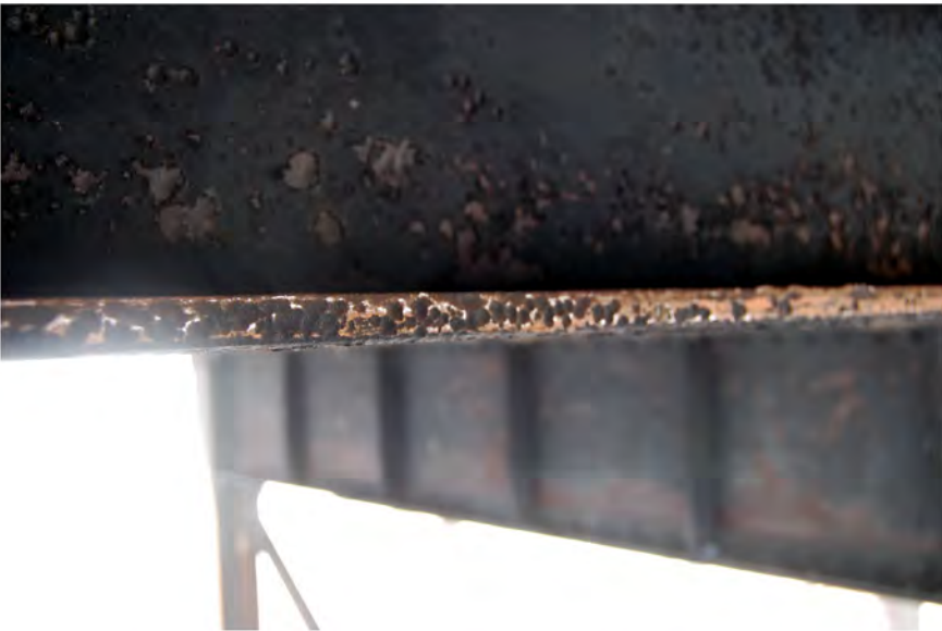
RUST PITTING OF BOTTOM FLANGE
