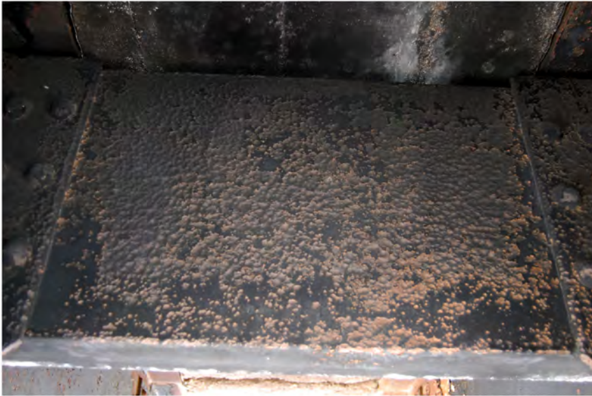
RUST PITTING OF DIAPHRAGM
