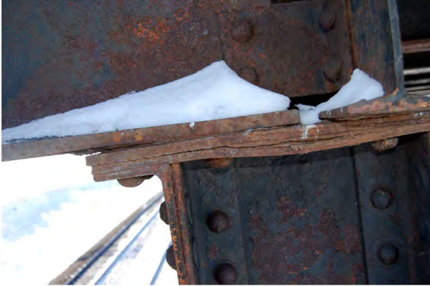
PACK RUST AT BENT/GIRDER CONNECTION
