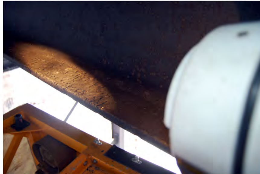
SECTION LOSS TO TOP OF BOTTOM FLANGE OF CENTER SPAN GIRDER
