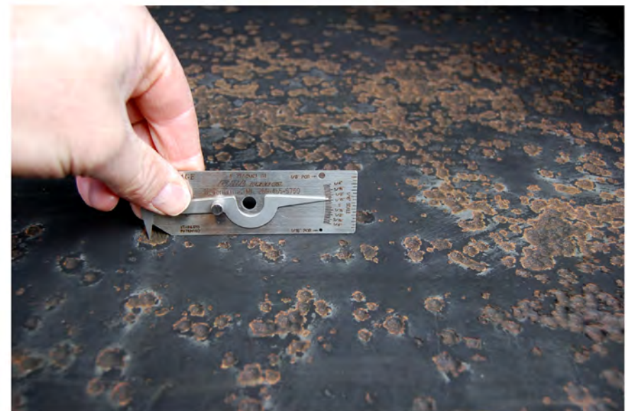
RUST PITTING 1/16" DEEP
