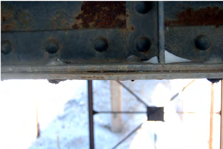
PACK RUST OF COVER PLATE SOUTH BENT CAP
