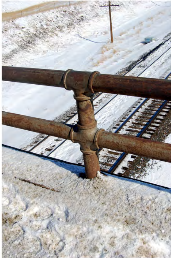
COLLISION DAMAGED RAIL POST
