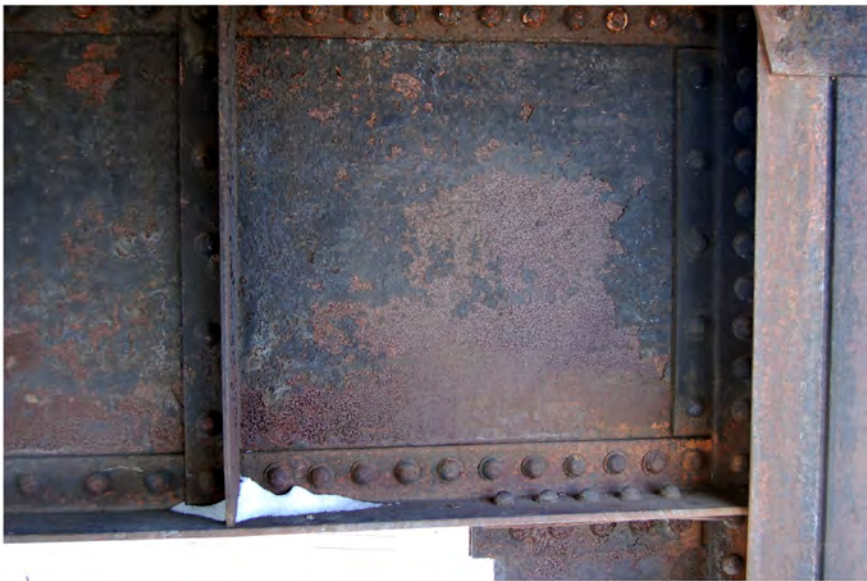
RUST ON BENT CAP
