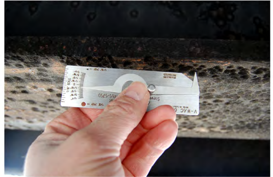
RUST PITTING OF BOTTOM FLANGE
