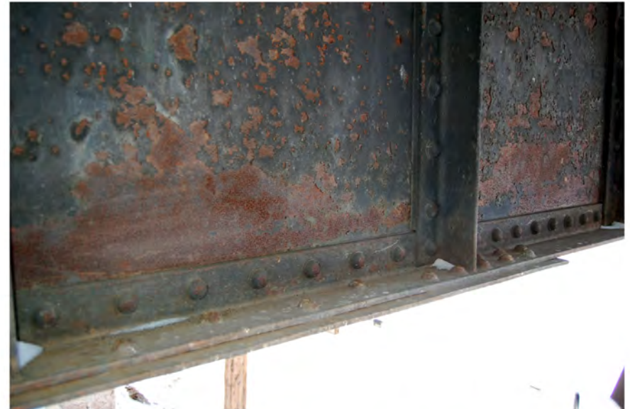
RUST ON NORTH BENT CAP
