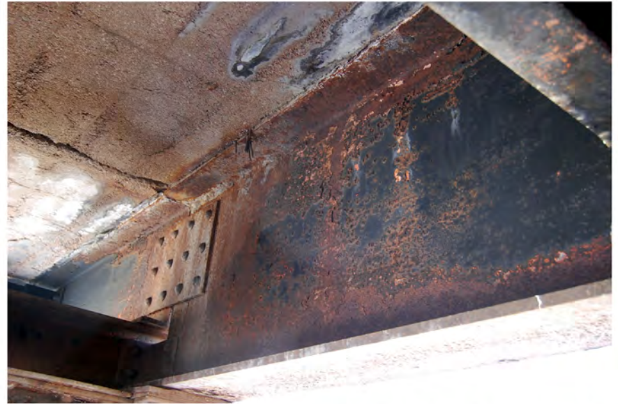
RUST ON GIRDER ENDS UNDER DECK JOINTS
