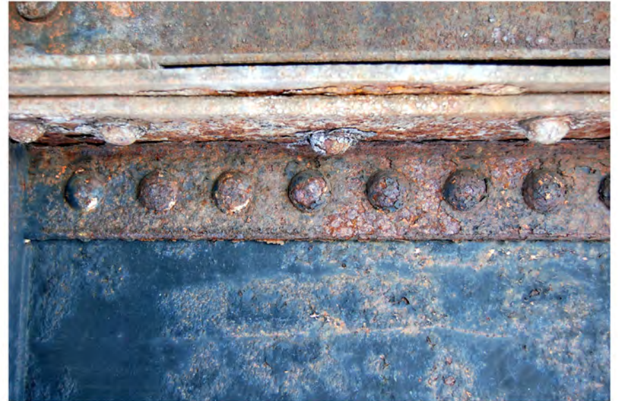
SECTION LOSS TO TOP FLANGE OF BENT CAP
