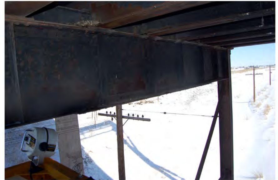
RUST ON NORTH BENT CAP
