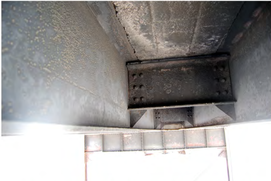
GIRDER AND DIAPHRAGMS PITTING IN CENTER SPAN
